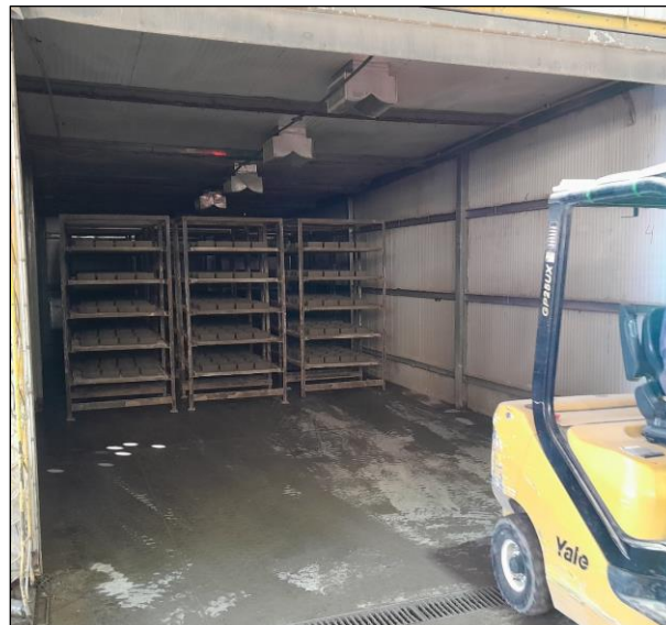
FIGURE 6: STEAM CURING CHAMBER
