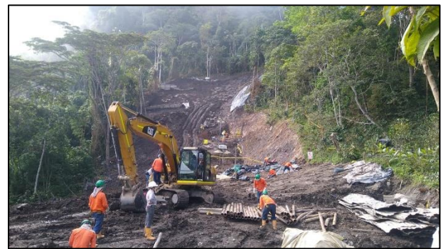
FIGURE 20: IN THE CENTRAL PART OF THE IMAGE, ESCARPMENT GENERATED DURING GROUND MOVEMENT WHEN THE SLOPE IS DECONFINED BY EXCAVATION.
