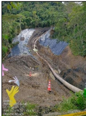
FIGURE 19: AERIAL PHOTOGRAPH OF THE PIPE EXCAVATION PROCESS CARRIED OUT AT CASE STUDY SITE 2.
