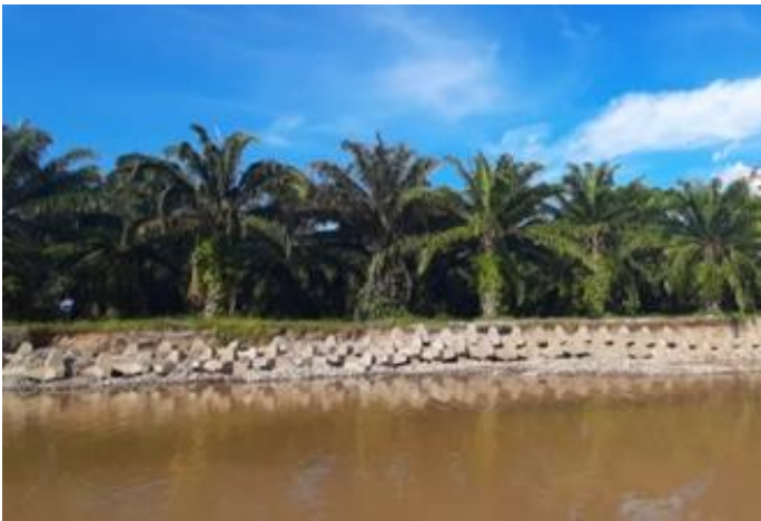
FIGURE 2. Riverine defense with concrete blocks. Source: Internet (2020). Current breakers are drainage works applied to the management of surface waters, which are built perpendicular to the line of maximum slope of the right-of-way, in order to capture and evacuate runoff water out of it and prevent it from making extensive routes. where the surface of the land is unprotected.
