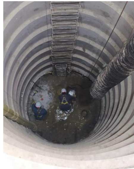
FIGURE 4. Horizontal drain capture chamber for piezometric level abatement. Source: Internet (2020). Water flows into the well from horizontal perforated tubes, with the water being pumped out. Drains can be drilled with some upward inclination to penetrate more than one aquifer horizon. These drains are placed using pneumatic hammers or by injection. The length of the drains varies depending on the area to be drained, and can vary from 30 to 100 m in length.
