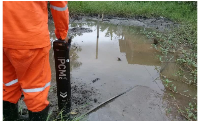
FIGURE 5: PIPELINE POSITION MAPPING USING PCM EQUIPMENT AND METHODOLOGY
