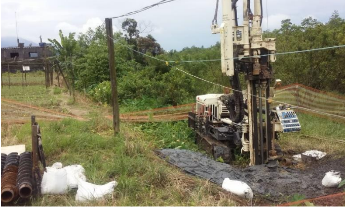
FIGURE 9: INTEGRATED GEOTECHNICAL INVESTIGATION EMPLOYING SPT (STANDARD PENETRATION TEST) AND ROTARY DRILLING TECHNIQUES.
