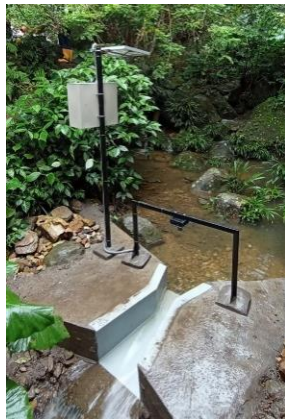
FIGURE 15: AUTOMATED MONITORING SYSTEM OF SURFACE WATER SOURCES THROUGH PARSHALL-TYPE FLUME
