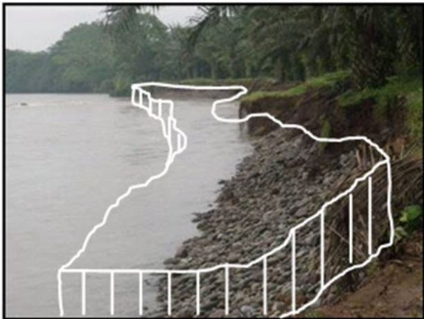
Figure 1: Magnitude of erosion with a loss of the left bank in 20m.
