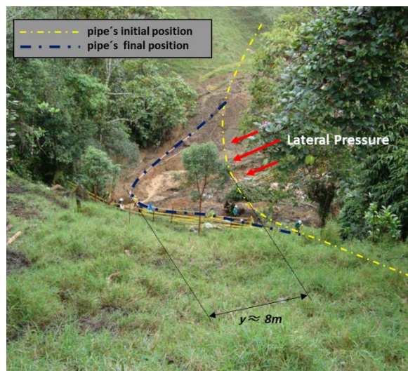
FIGURE1 DISPLACEMENT OF A PIPE DUE TO THE EFFECT OF THE AVALANCHE
