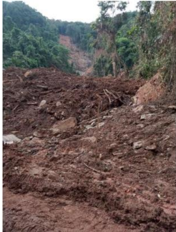
Figure 1: km 36+150 right after the rainfall (4)
