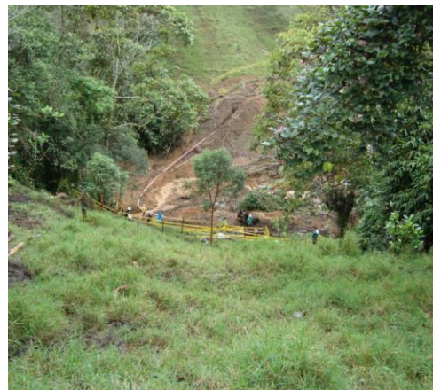
FIGURE 9 DISPLACEMENT OF THE PIPE, DUE TO AN INSTABILITY PROCESS.
