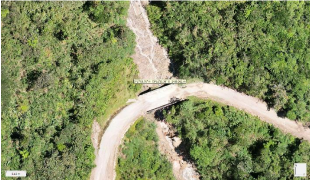
FIGURE 8: Monitoring of the crossing place with UAV's technique. The mass was 0,9m under the plate of the bridge. September 2023. Source: OCENSA.
