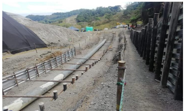
FIGURE 5: EXCAVATION FOR STRESS RELIEF.
